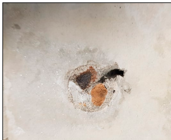
Figure 9. Concrete fracture outside the notch.
