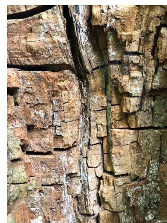
Figure 3.1. An image showing the cubical structure of red rotten wood.
