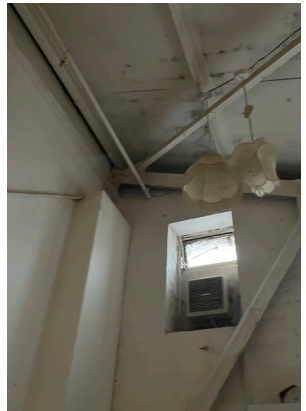
Partly blocked window
