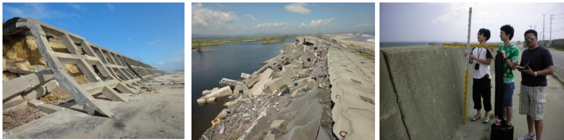
Figure 1. Failure of coastal dykes and the field survey team of UEL-Waseda University research collaboration
