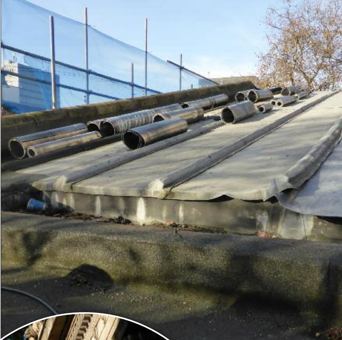
Starting the Portico leadwork – over-length lead bays, asphalt and cement. Note the two fixing holes to the antefix, bottom left
