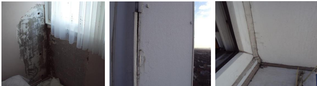
Figure 4. 10. Problems in Estate B (Source: Author).
