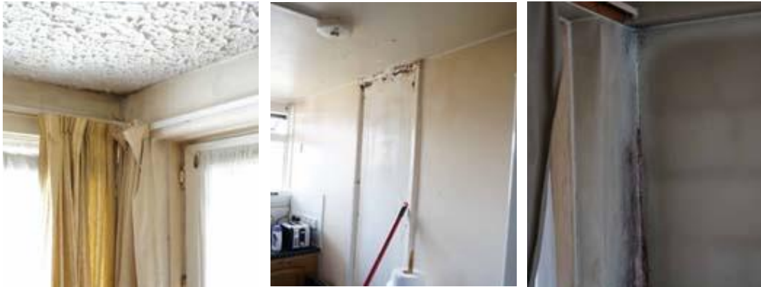
Figure 4. 5. Site investigation: mould issue at Estate A (Source: Author).
