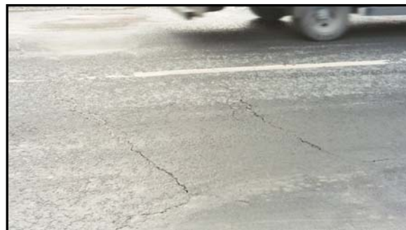
Figure 1. Subsidence cracks, parallel to trench walls on the surface
