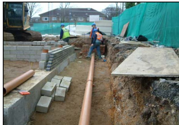
Figure 6. Two length of pipe connecting manhole without construction Joint at the interface
