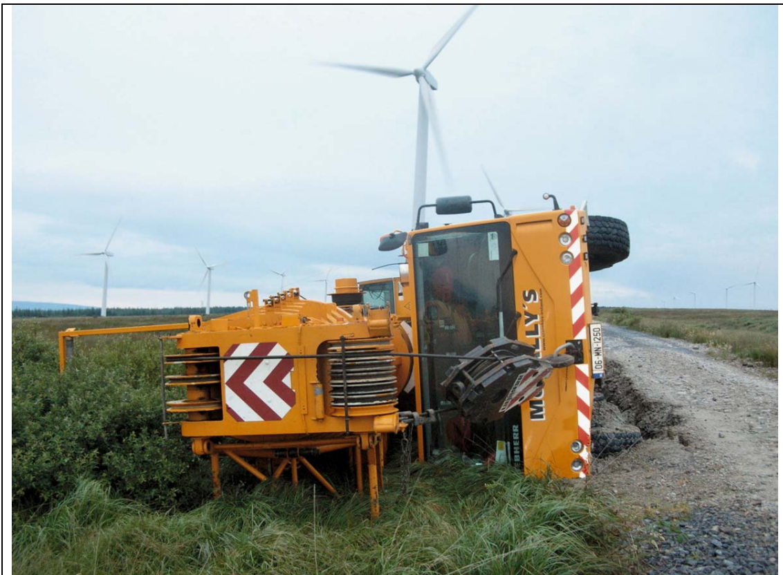
Figure 4. Crane accident arising from failure of floating road.
