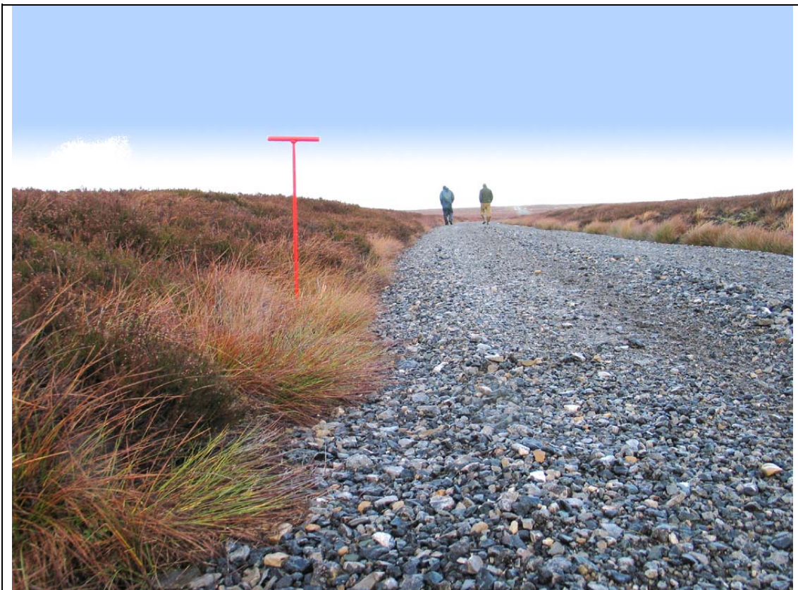
Figure 3. Floating road with evidence of sinking.
