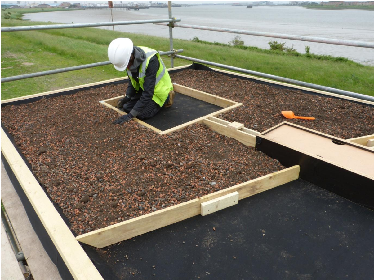
Figure 16. Installation of aggregates on the Phase 2 green roof experiment at Barking Riverside, East London. The aggregate volume on all roofs was measure so as to be as identical as possible. Placement of mounds was done using a wooden frame template for reproducibility. The only thing that varied between green roofs was the east-west orientation of the two substrates.
