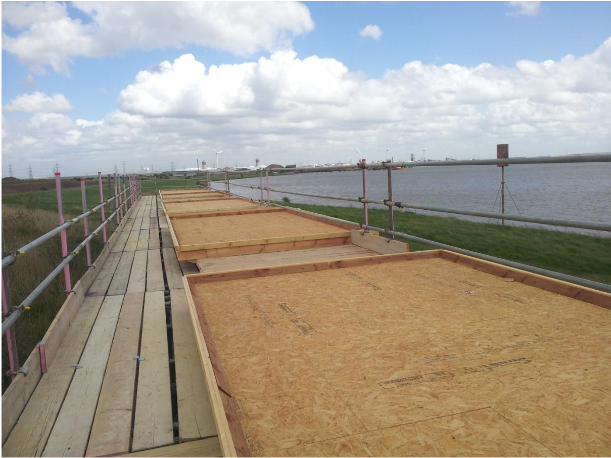
Figure 12. Completed wooden bases for the Phase 2 green roof experiment at Barking Riverside, East London. Frames were based on the Green Roof Shelter Company's designs ( www.greenroofshelters.co.uk ).
