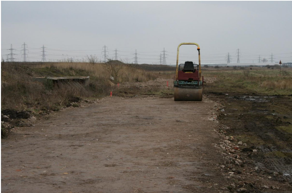
Figure 7. Construction of a levelled area on which the container bases for the Phase 2 green roof experimental treatments could be sited at Barking Riverside, East London. The area in question was to the rear of the seawall pathway.
