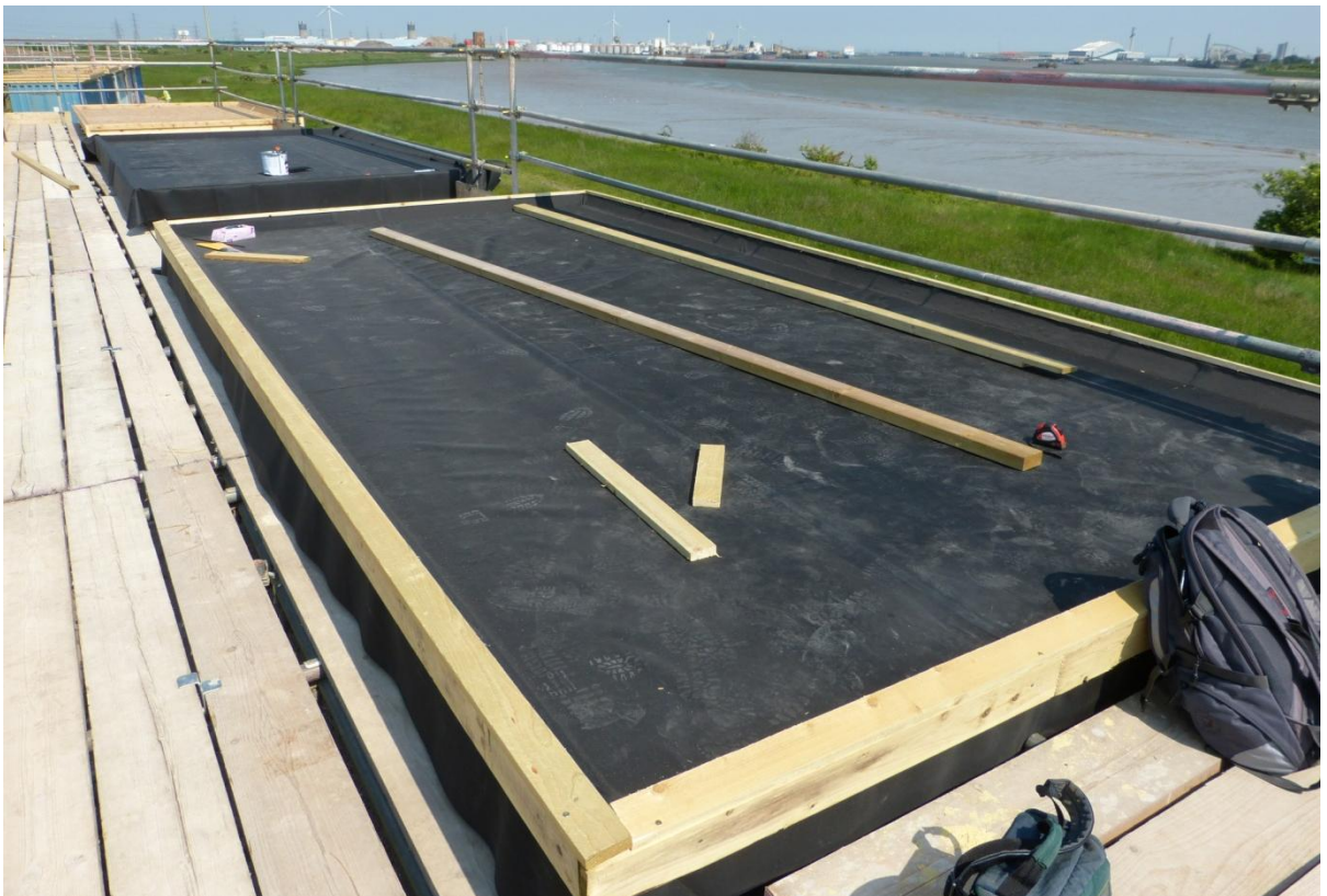
Figure 14. Installing the Hertalan EPDM water proofing membrane on the Phase 2 green roof experiment at Barking Riverside, East London. The membranes were supplied by Hertalan ( www.hertalan.co.uk ) in support of the research.
