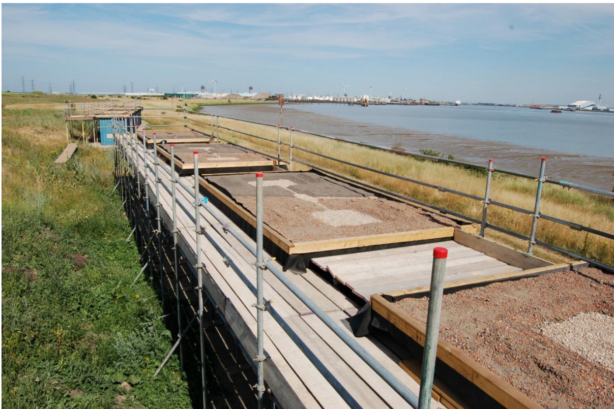
Figure 16. Completed construction of the Phase 2 green roof experiment at Barking Riverside, East London. Image shows the layout of all 9 green roof test platform surrounded by edge protection scaffold.
