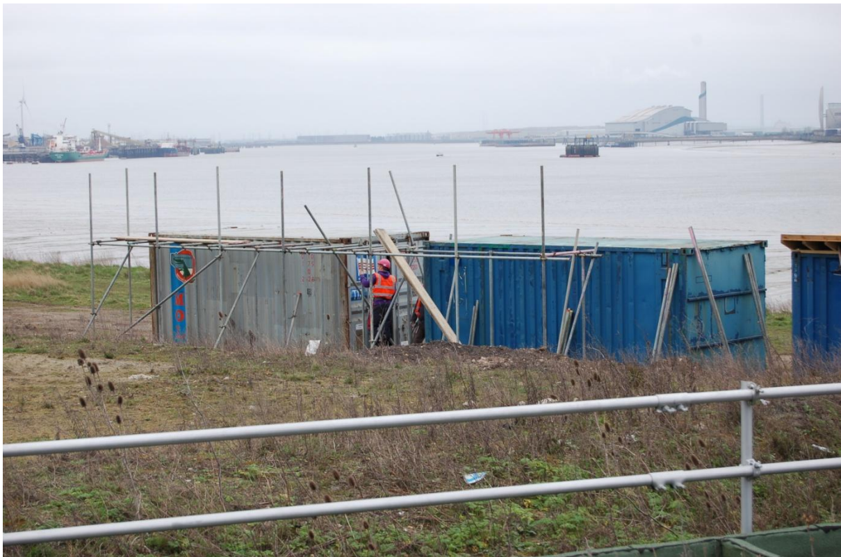
Figure 10. Edge protection scaffolding being erected for the Phase 2 green roof experiment at Barking Riverside, East London. The scaffold will remain in place for the duration of the experiment.
