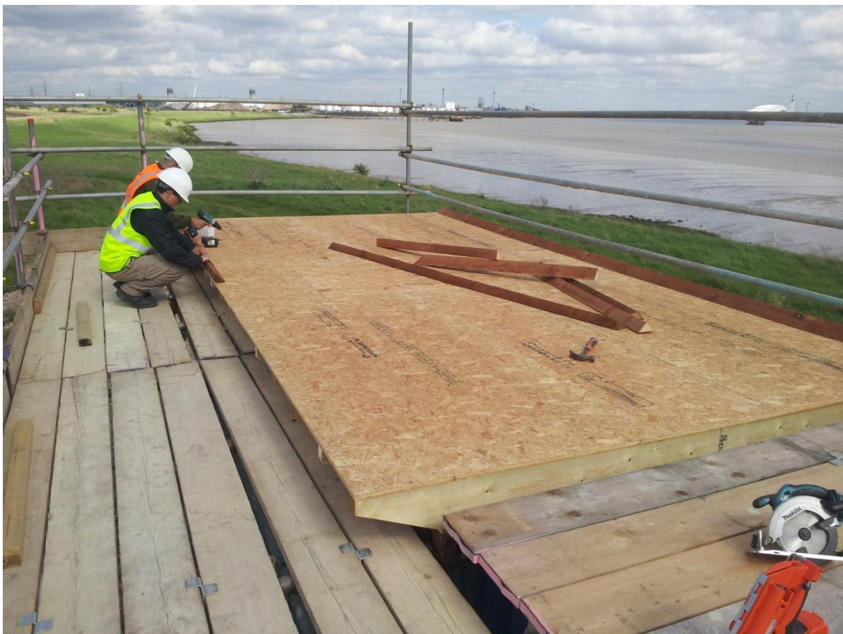
Figure 11. Construction of the wooden bases for the Phase 2 green roof experiment at Barking Riverside, East London. Frames were based on the Green Roof Shelter Company's designs ( www.greenroofshelters.co.uk ).
