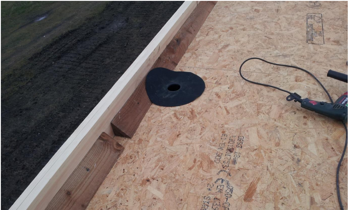
Figure 13. Drainage outlet installed for the Phase 2 green roof experiment at Barking Riverside, East London. A single drainage outlet was installed for each green roof.
