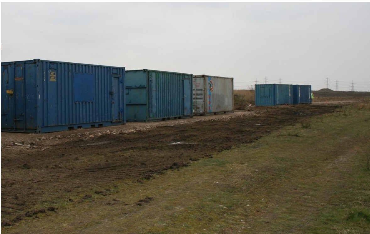
Figure 9. Five freight containers in place for the Phase 2 green roof experiment at Barking Riverside, East London. Gaps between freight containers are designed to create and 'ecological gap' between green roof experiments (gaps were at least 2 metres wide).
